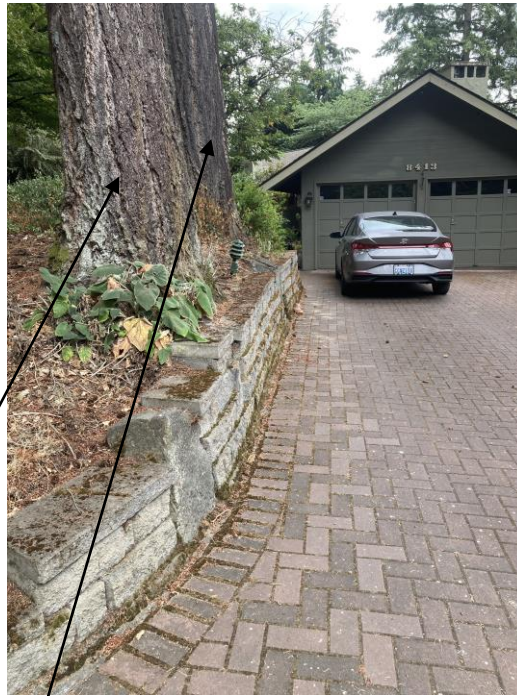
Tree No. 3 and 4 growing atop block retaining wall
